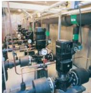
Figure 7: Engine room with eight pumps
