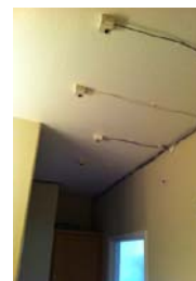
(a) Sensor Installation
