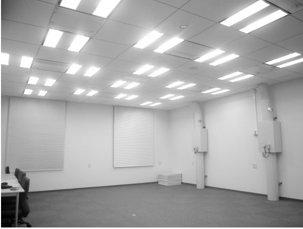
Fig. 1. Laboratory Equipped with a Networked Lighting System
