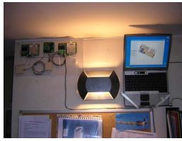
Figure 4- The local station is fitted on the wall in the nurse office
